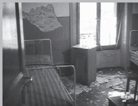
Shelter would need to be provided for thousands to tens of thousands of people who do not know if their homes are still habitable. Imagine your aunt had been sleeping here.
